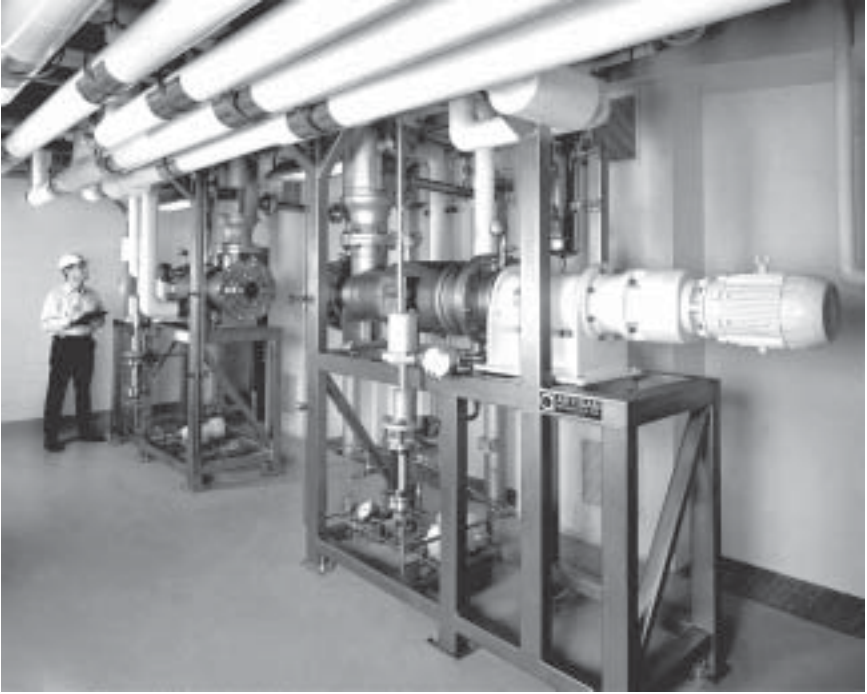
Installed in a cGMP facility, this Rototherm is designed to manage solvents and to purify API, intermediates or fine chemicals.
